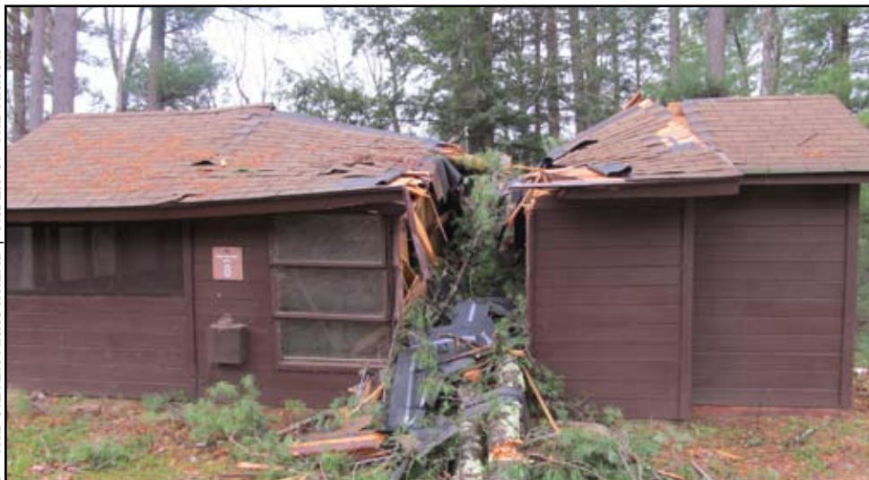
Hurricane Sandy damage at the Ten Mile River Scout Reservation operated by the Greater New York Councils.
